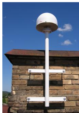
Fig. 6 Mount of antenna in base station Madona
