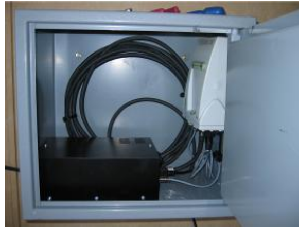
Fig. 7 Base station equipment
