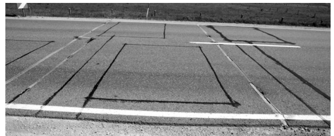
Fig.1. Installed piezoelectric WIM sensors and inductive loops.
