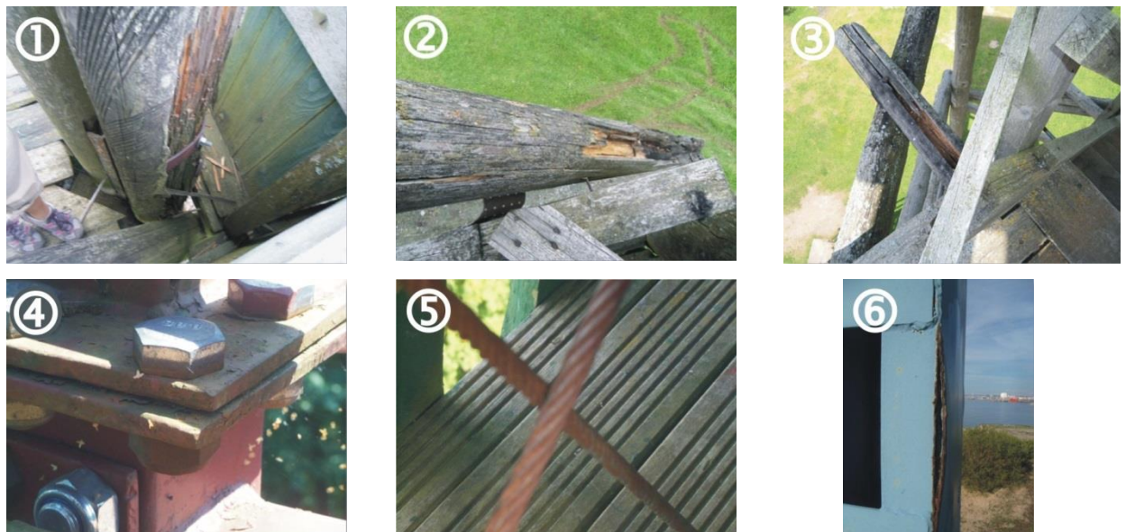
Figure 3.3. Typical damage of timber (1-3) and steel (4-5) observation towers
