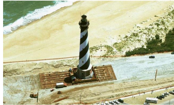
Figure 35. Cape Hatteras Lighthouse, Dexter Stetson, The United States [Photo by WJE Projects, Annex 7].
