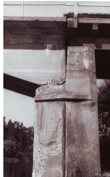
Fig.8. Pier before repair in 1985
