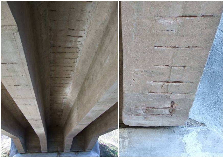
Fig.9. Spalling of the concrete due to insufficient concrete cover and corrosion of reinforcement
