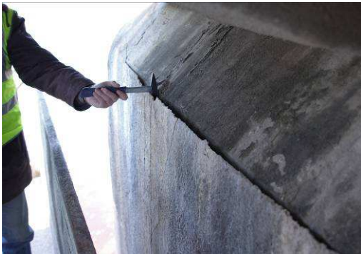
Fig.6. Delimitation of shotcrete layer of pier positioned below faulty expansion joint
