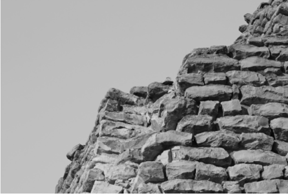
Fig. 3. Characteristic quality of the blocks laid in the lower part of the Step Pyramid (southern façade).
