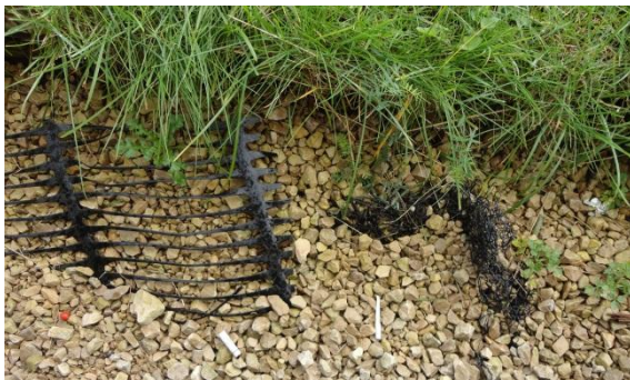
Figure 7. Geotextile sticking out from gravel (Source: photo by the authors, 2012)
