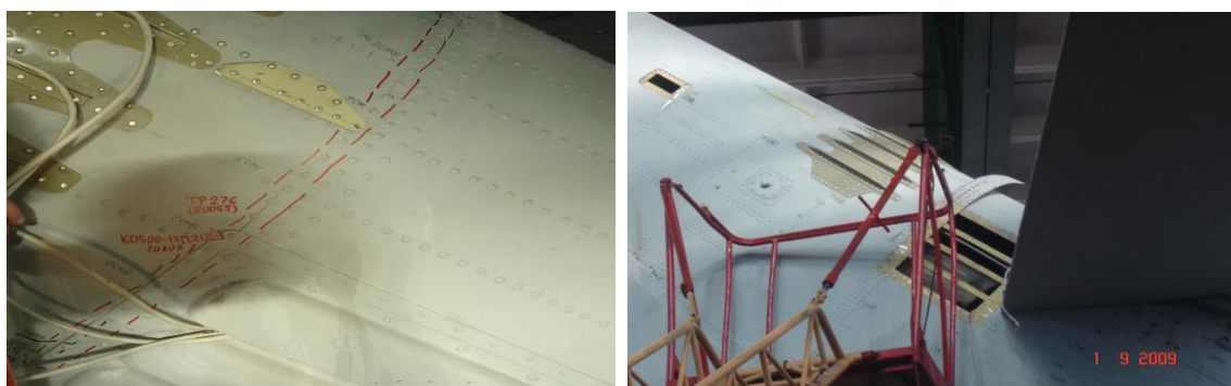
Fig.5.12 Fatigue crack under splice plate of air-blow-off louver.
