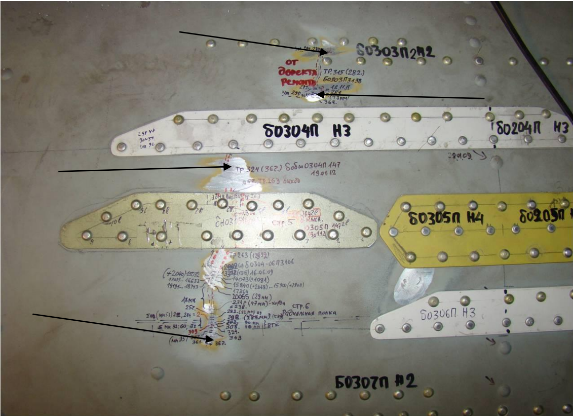
Fig.5.16 Three fatigue cracks that emergences under repair pads and new one. It is clear seen how three fatigue cracks have to coalesce to one mainline crack.
