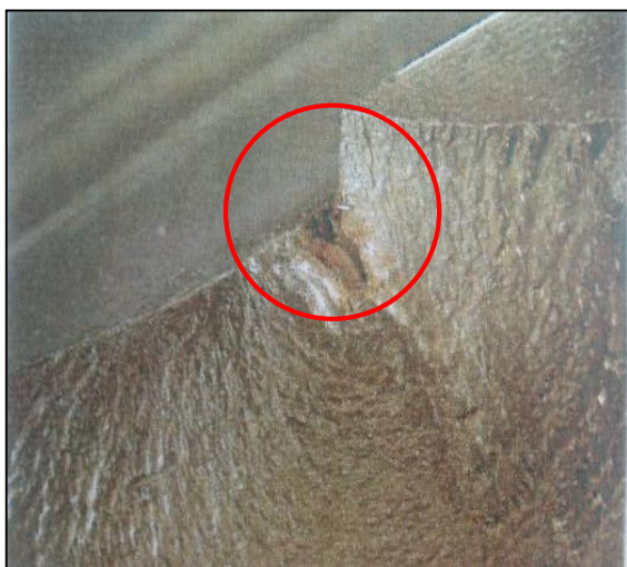
Fig.6. Enlarged picture of the crack starting point
