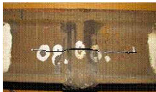
Fig.2. View of a thermic weld score and cracks revealed.
