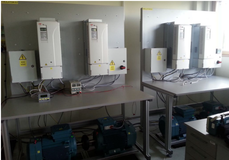
Fig. 3.6. DC power flow emulators developed in the RTU AREUS demo laboratory.
