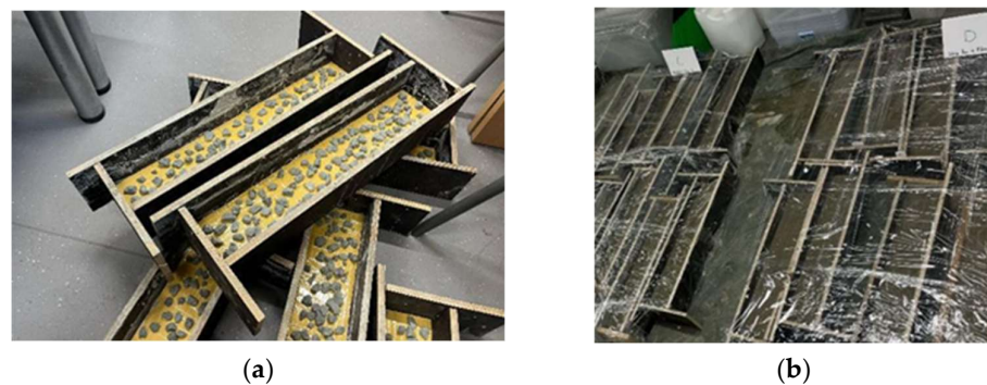
Figure 3. Production of the group A specimens: (a) placement of specimens in the moulds; (b) filling of the moulds with concrete.
